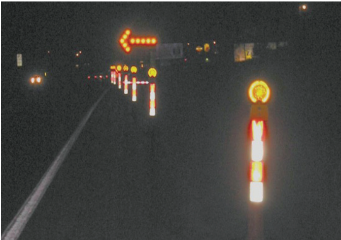
Figure 7. Sequential Warning Lights at a Work Zone (43)
